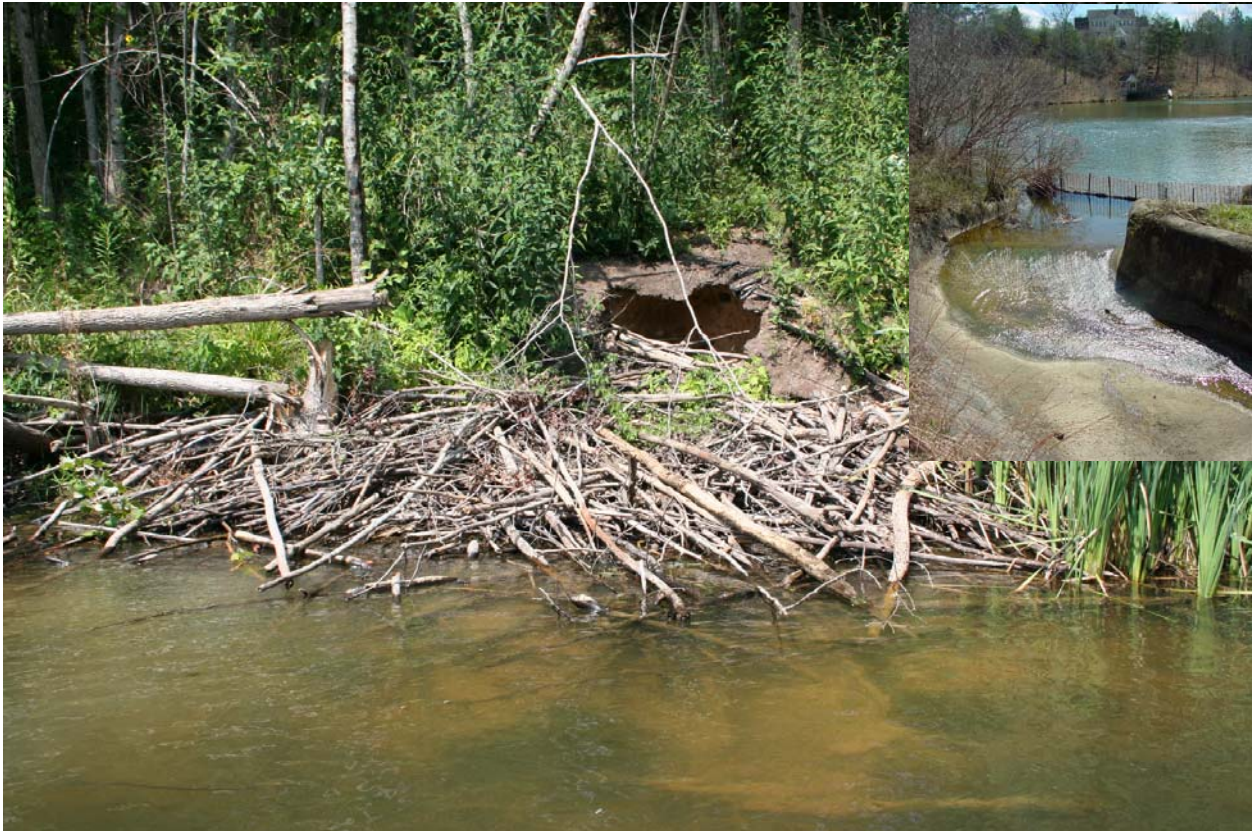
Beavers and muskrats can bore in to the side of the dam and weaken its structure. Emergency spillways should be lined with concrete if they receive heavy flow (inset).
