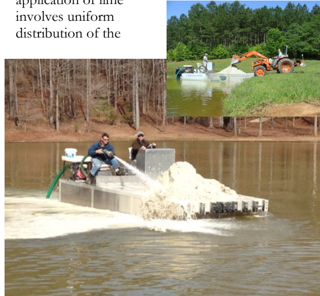
Bulk lime is applied by washing it directly into the water in such a way that it covers most of the lake bottom.
